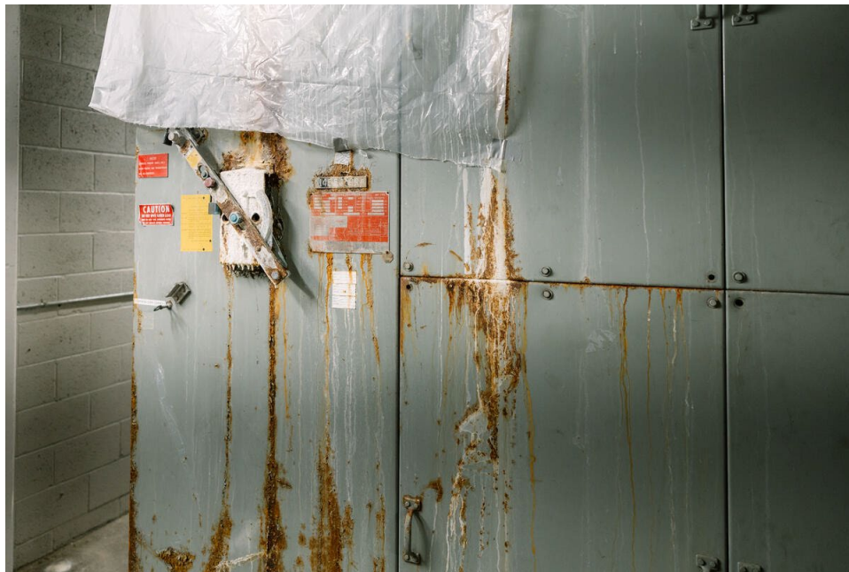
Water damage in the electrical vault, one of many projects that will be addressed.
